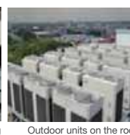
Outdoor units on the roof
